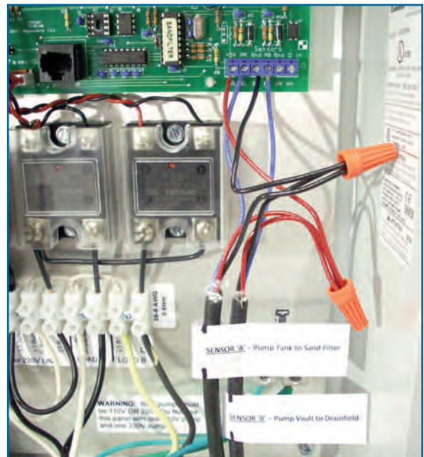
Figure 8: Sand Filter Panel
